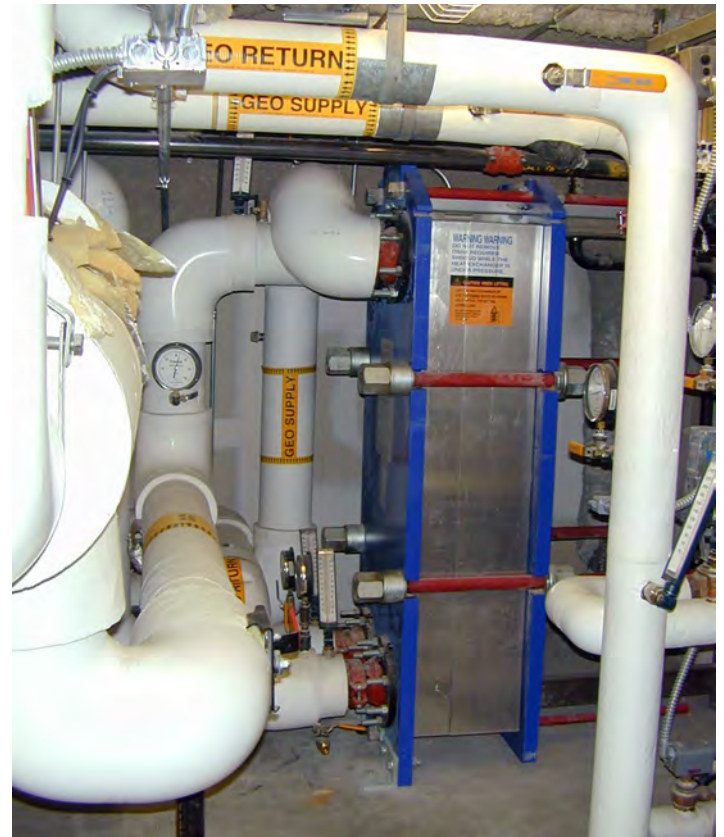
A plate heat exchanger connecting the heating system of the Elks Rehabilitation Hospital in Boise, Idaho to the city's geothermal district heating system. Photo credit: Bruce Green/NREL
