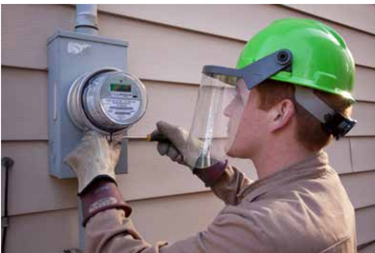
Smart meter installation. Credit: Portland General
