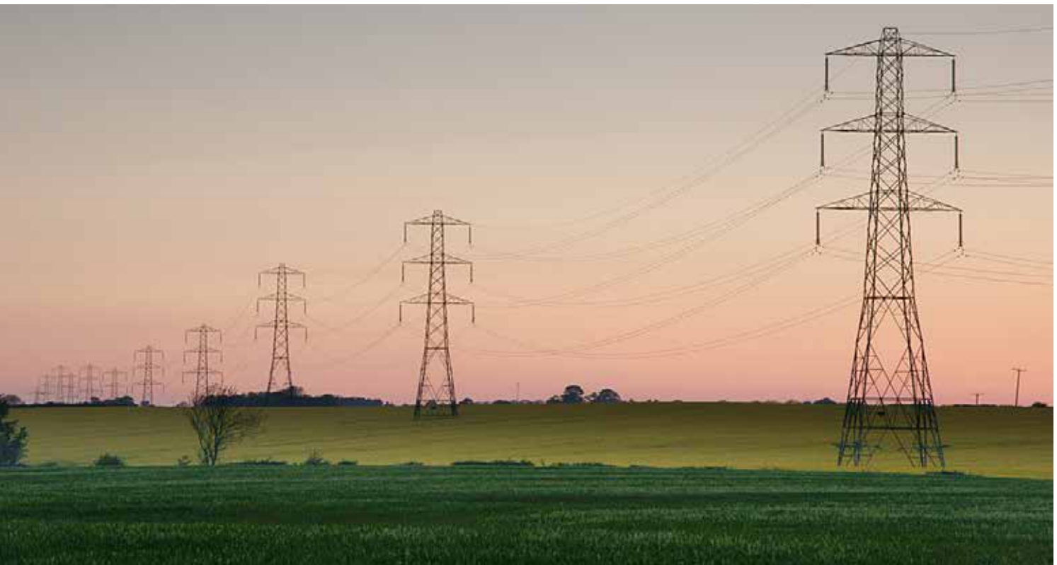
Transmission lines. Credit: Ian Britton
